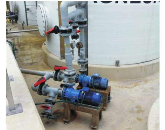
Transfer of Hydrofluoric Acid, Nitric Acid and Phosphoric Acid in a Germany based Fine Chemical Plant
